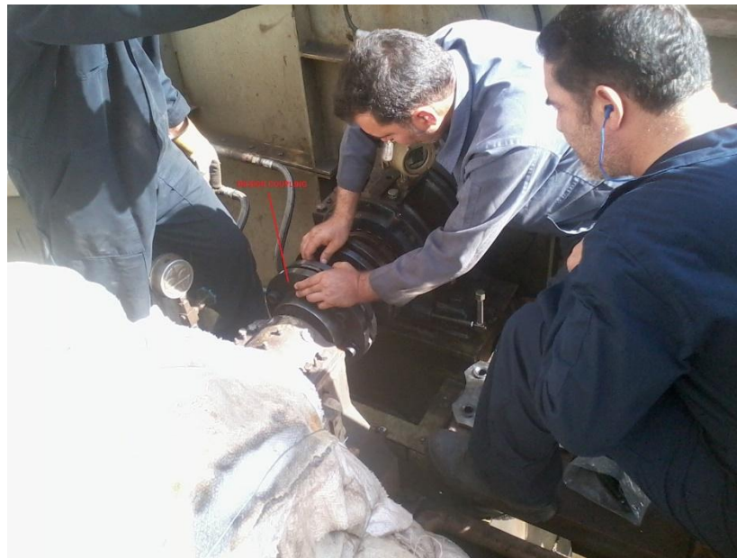
COUPLING ASSEMBLED BY OPERATOR BETWEEN TURBINE AND BLOWER
